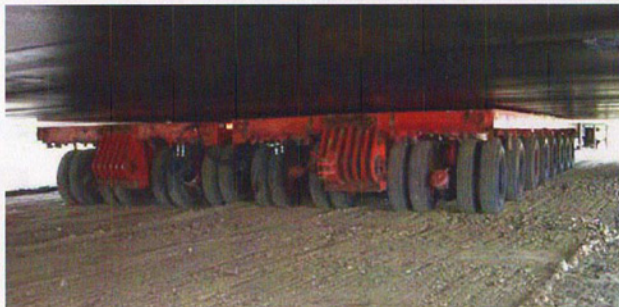
Two 8-line and two 6-line hydraulic platform trailers were joined laterally and positioned under the rear and front sections of the barge.
